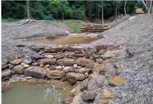
Source: Anne Arundel County – Design Guidelines for Step Pool Stormwater Conveyance (SPSC) Systems, May 2022
