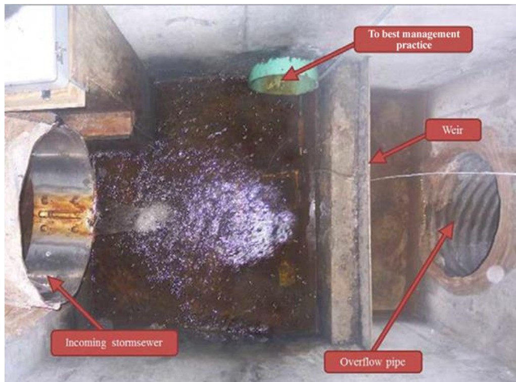
Figure 2.8-3 - A commonly used flow bypass structure configuration that bypasses flow when the capacity of the outlet pipe supplying the BMP is exceeded (photo courtesy of NCSU-BAE)
