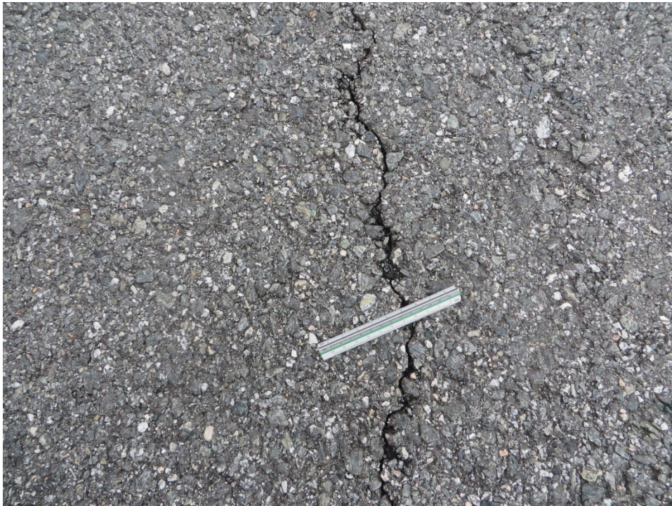
A01NH-10. L&T Cracking (Sample Unit No. 02).
