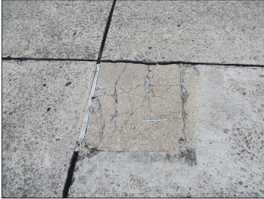
FIGURE H-14 HIGH-SEVERITY PATCHING
