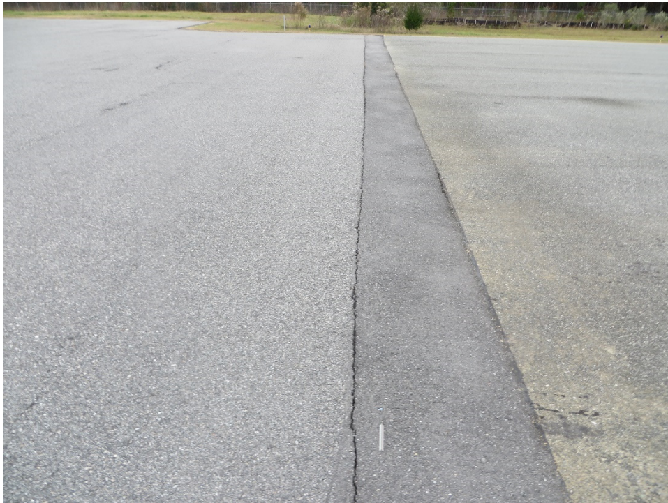
A01NH-20. Patching (Sample Unit No. 01).
