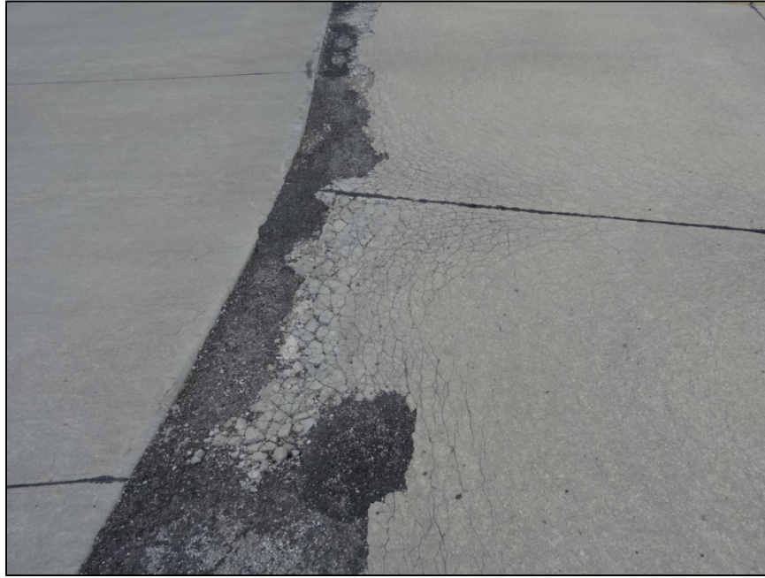
FIGURE H-13 HIGH-SEVERITY DURABILITY CRACKING
