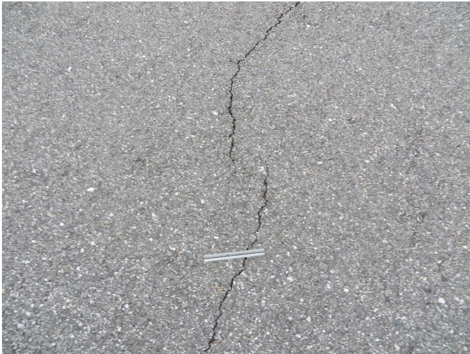
R119NH-10. L&T Cracking (Sample Unit No. 05).
