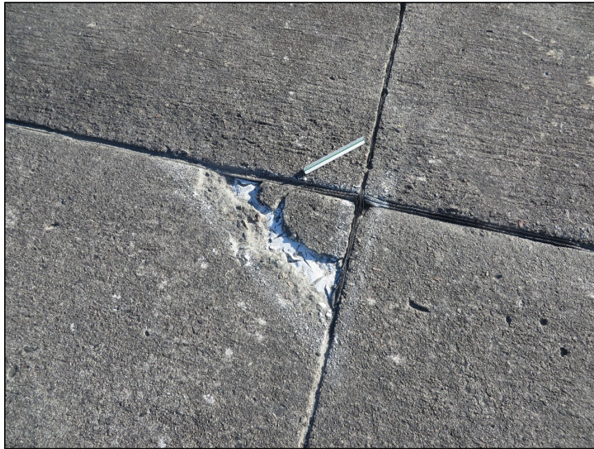
FIGURE H-19 HIGH-SEVERITY CORNER SPALLING
