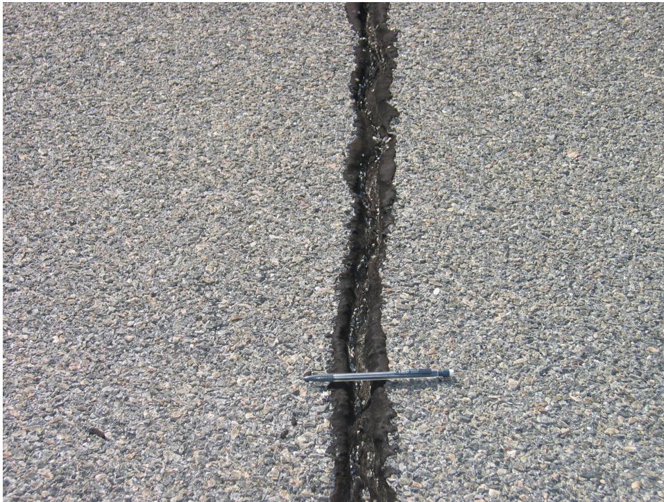
R119NH-10. L&T cracking.
