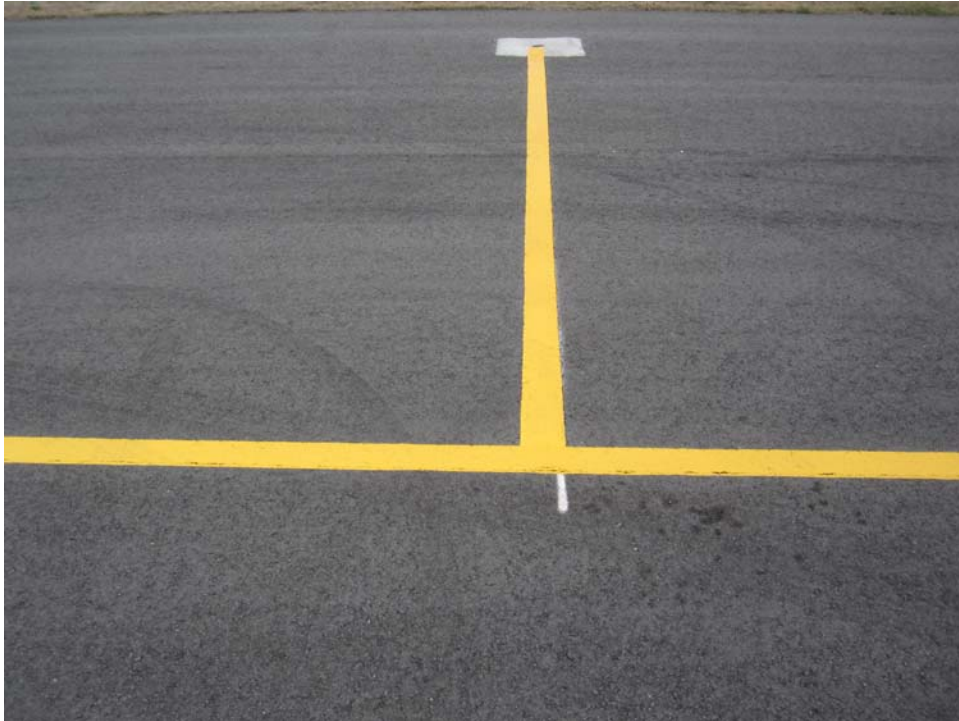
A01JS-10. Satisfactory Paint.
