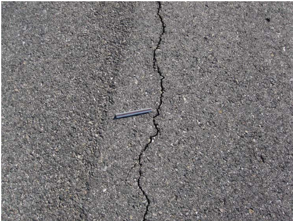
R1129JS-10. Longitudinal and Transverse Cracking (Sample Unit #03).
