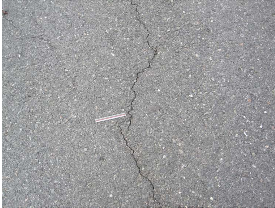
THANGJS-10. Longitudinal and Transverse Cracking (Sample Unit #05).
