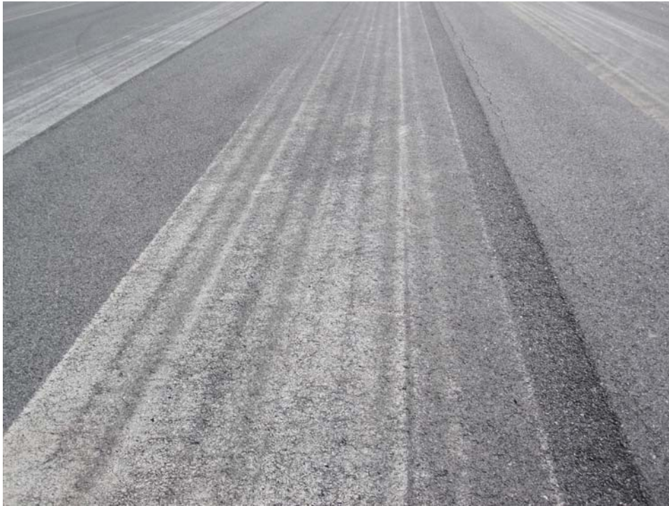
R1129JS-10. Unsatisfactory Paint.
