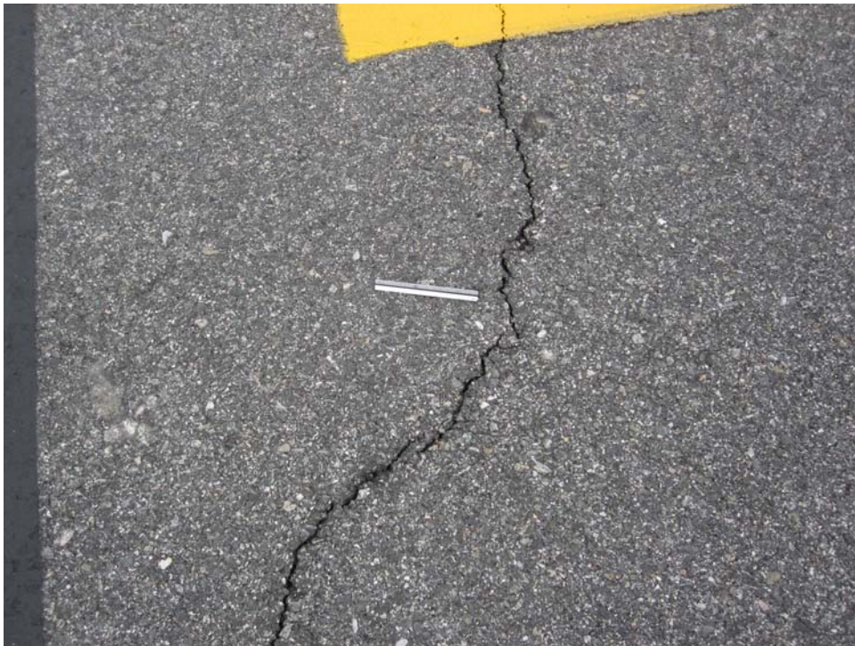
TAJS-10. Longitudinal and Transverse Cracking (Sample Unit #02).
