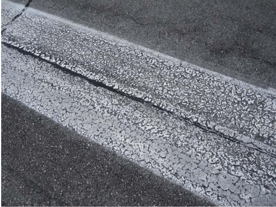
R523CH-10. Unsatisfactory Paint.
