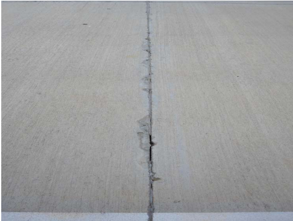
AHELICH-10. Joint Seal Damage (Sample Unit #01).
