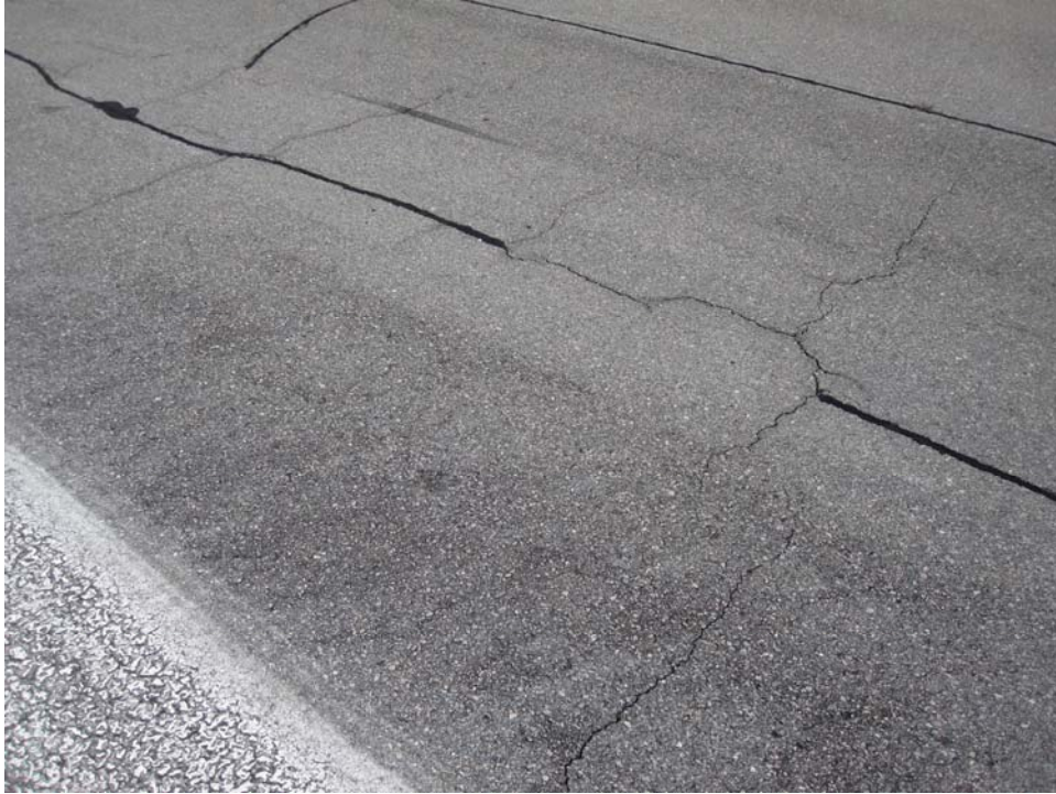
R523CH-10. Block Cracking (Sample Unit #07).
