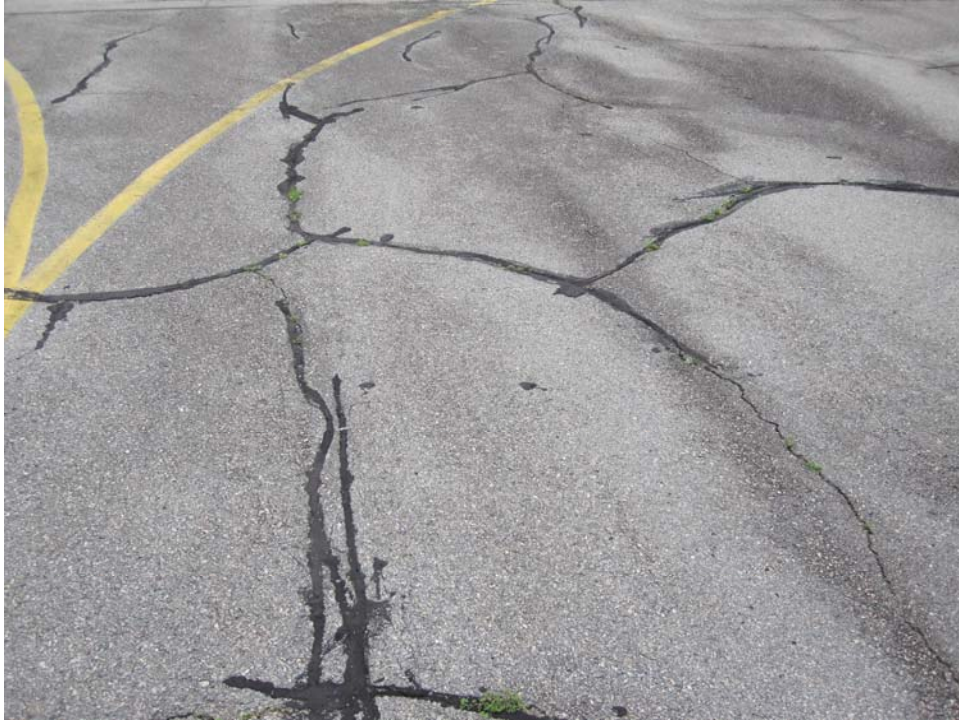
TACH-10. Block Cracking (Sample Unit #01).
