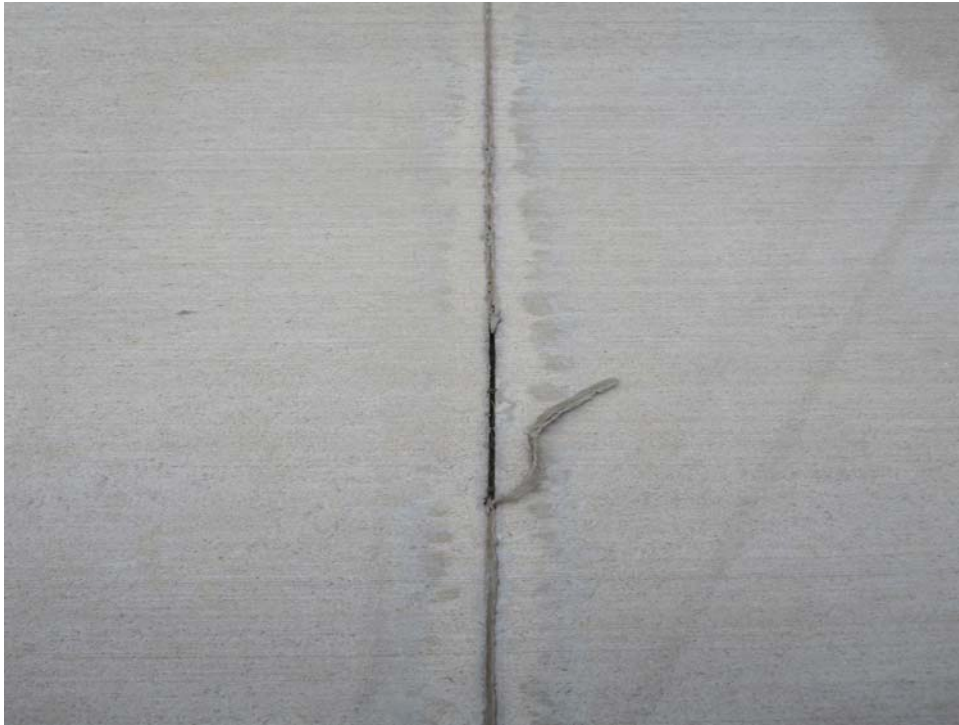
A01CH-30. Joint Seal Damage (Sample Unit #01).
