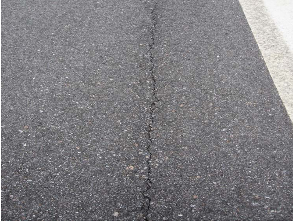
R1129CH-10. Longitudinal and Transverse Cracking (Sample Unit #03).
