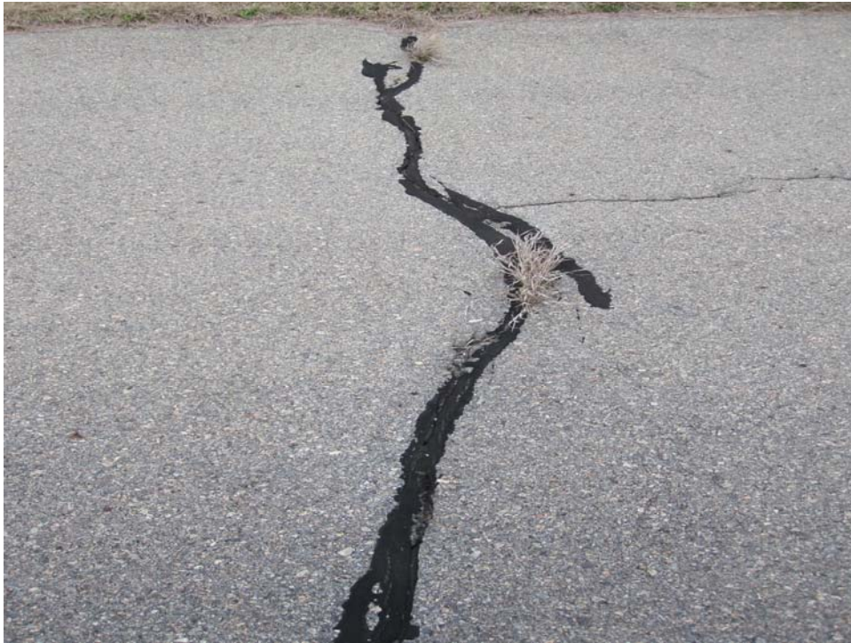
R523CH-10. Longitudinal and Transverse Cracking (Sample Unit #07).
