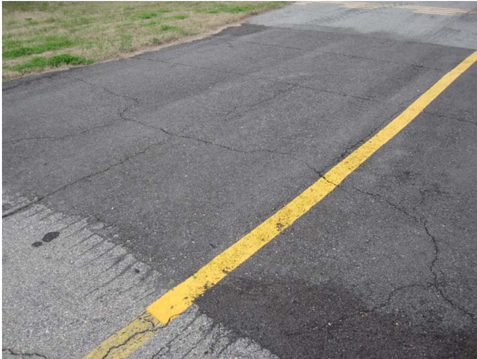
TACH-10. Patching (Sample Unit #01).
