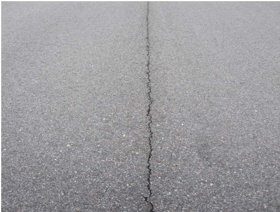
R1129CH-10. Longitudinal and Transverse Cracking (Sample Unit #11).
