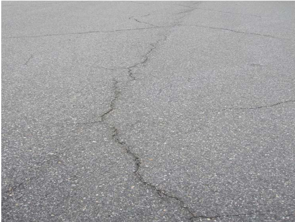
A01CH-10. Longitudinal and Transverse Cracking (Sample Unit #03).
