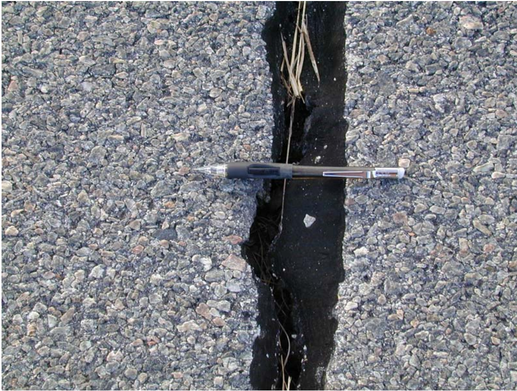
L&T cracking in section R119NH-10.
