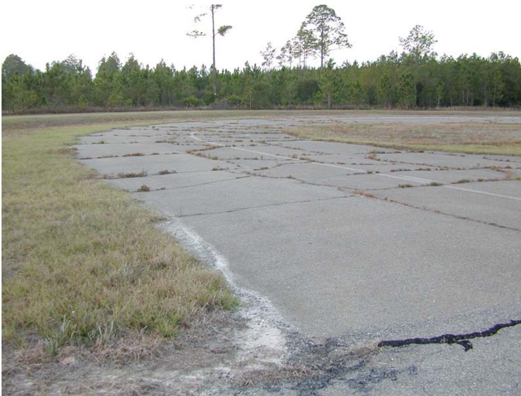
Overview of abandoned pavement in section R119NH-10.
