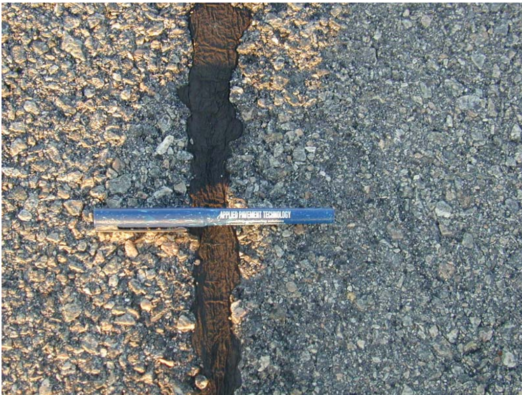
L&T cracking in section R523CH-10.
