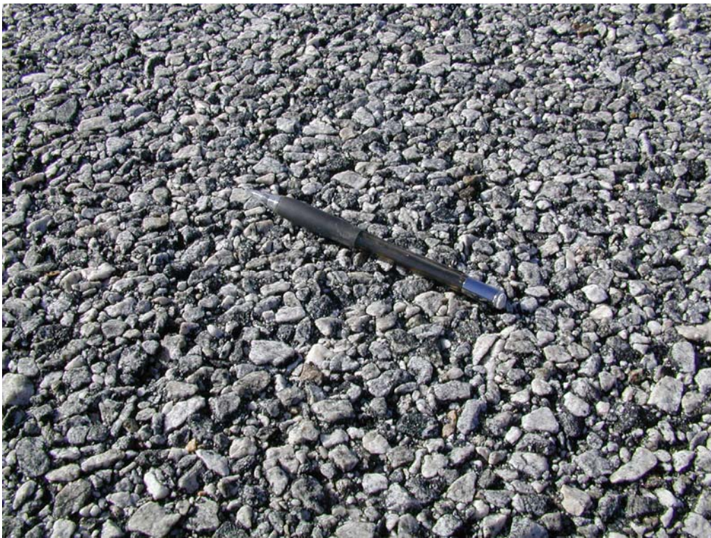
Raveling and weathering on section R1836JK-10.
