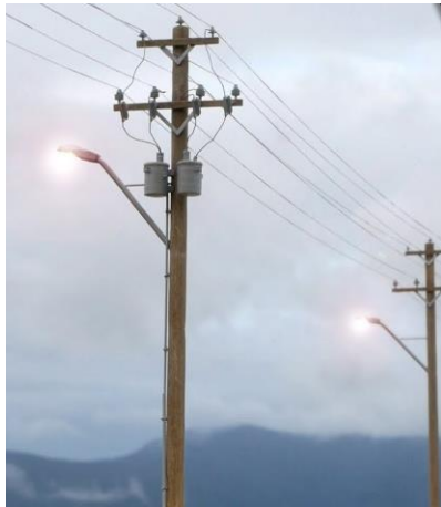
Low-cost lights on existing utility poles
