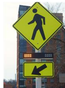
b: Rectangular Rapid Flashing Beacon (RRFB)
