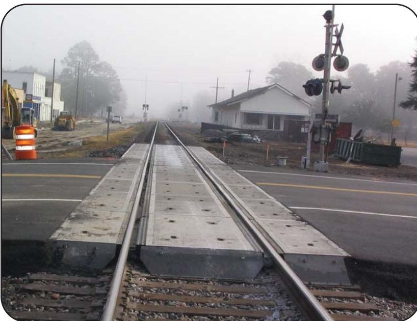
Among the accomplishments in FY 2004 are the construction of railroad crossings in Homerville, Clinch County. The above picture is Church Street on State Route 89.
