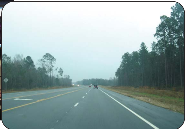
District Five performed 6.790 miles of widening for additional lanes on US 341 between Jesup and Odum.
